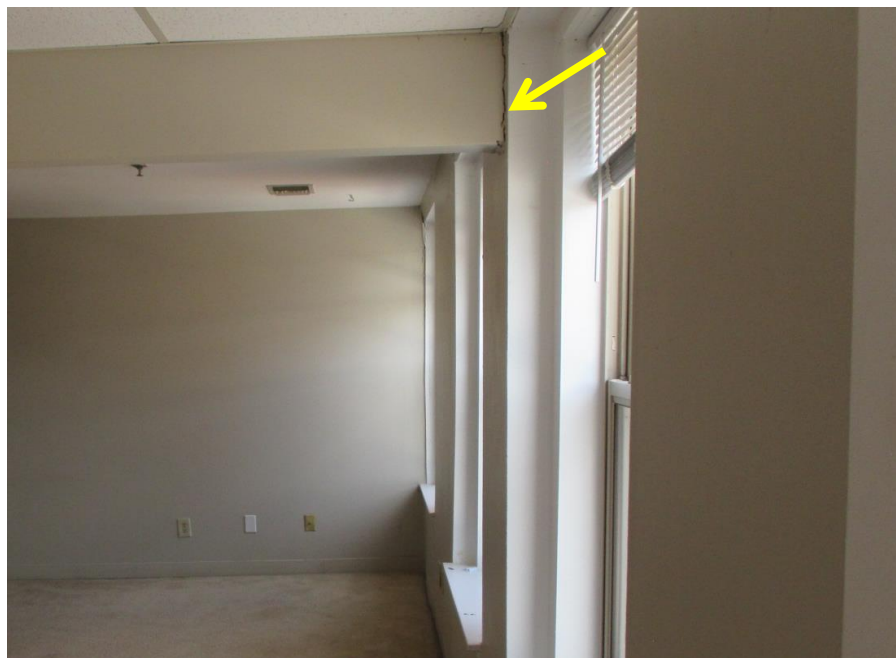
Photograph 30: Image from City file 20-7839. Note separation of gypsum board at beam to wall interface.
