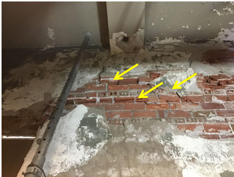
Photograph 12: February 2023 image from City file 23-6454. Note shear cracks and distress at interior masonry.
