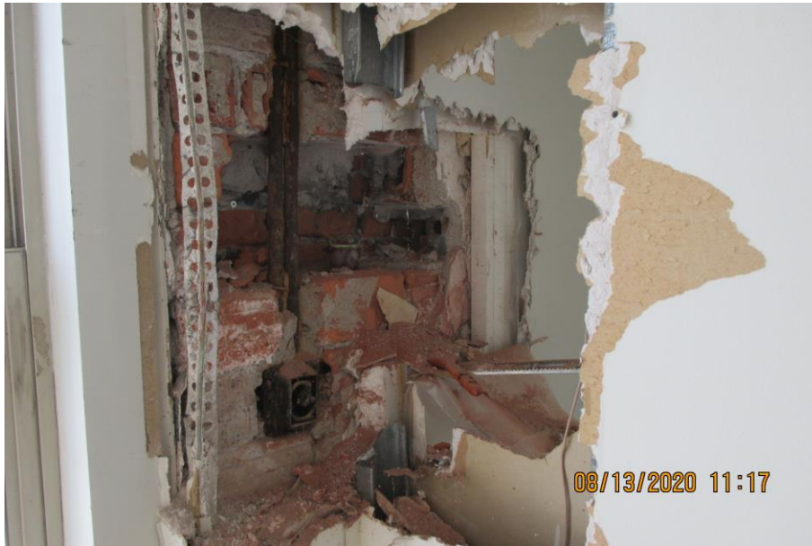
Photograph 7: August 2020 Image from City report. Note deterioration of brick masonry at interior wythes.
