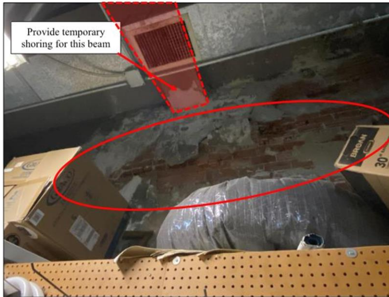
Photo 1 – Damaged Brick & Beam to Support
