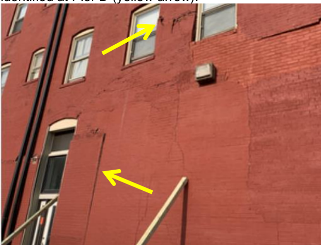
Overall view of portion of west elevation south of door. Note numerous areas of deterioration to wall.
