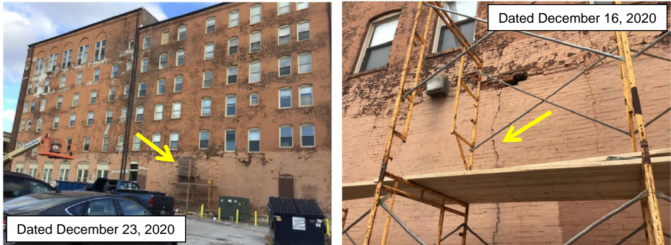
Fig. 28. West elevation photographs (Ref: City Reinspection Report, Task ID: 20-72033). Yellow arrow indicates crack in wall.
