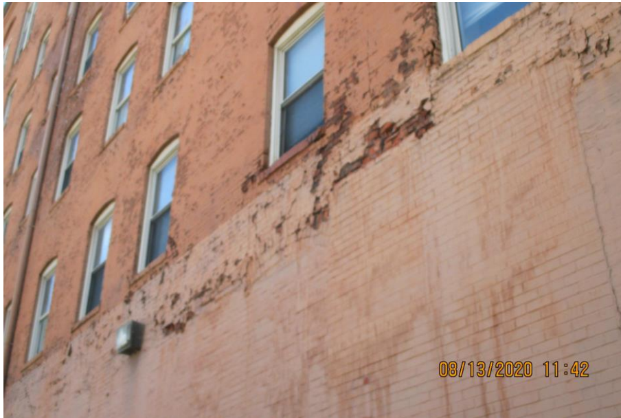
Photograph 3: August 2020 image of west elevation from City report. Note open mortar joints and masonry distress.
