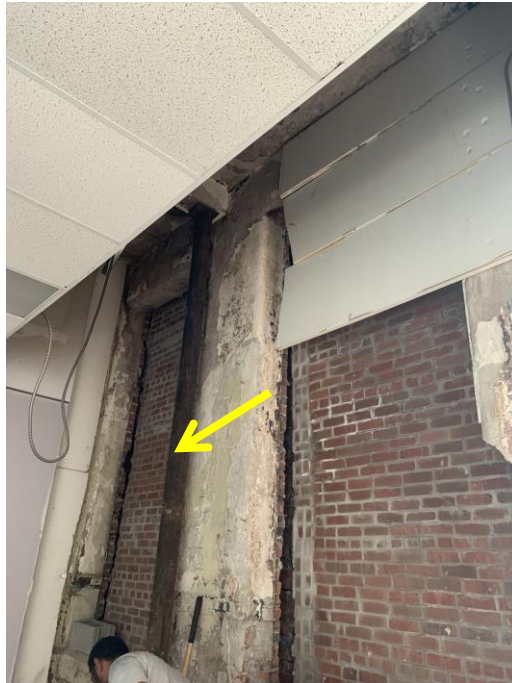
Photograph 31: Image from City file 23-30329. Note previously installed supplemental steel post.
