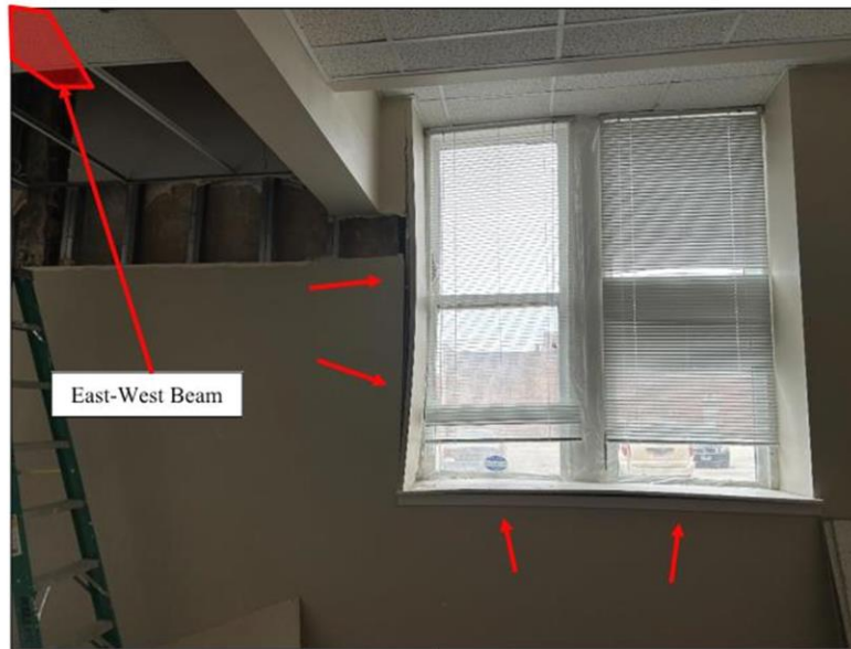
Photo 3 – Excessive Downward Pressure on Finishes
