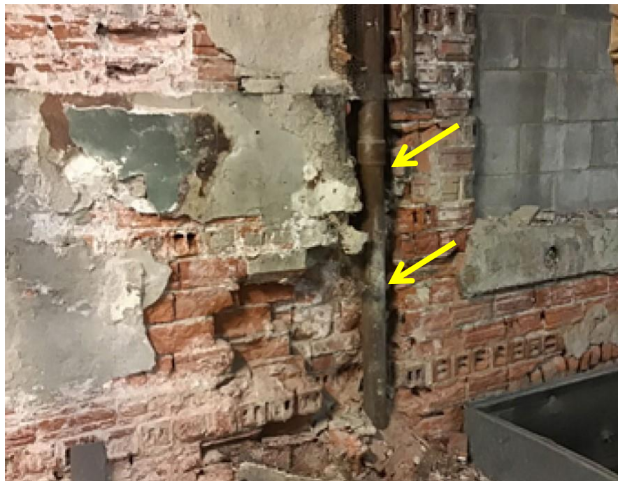
Photograph 24: Interior photo of west elevation wall from City file 23-6454. Note reduced wall thickness at location of plumbing embedded within wall.
