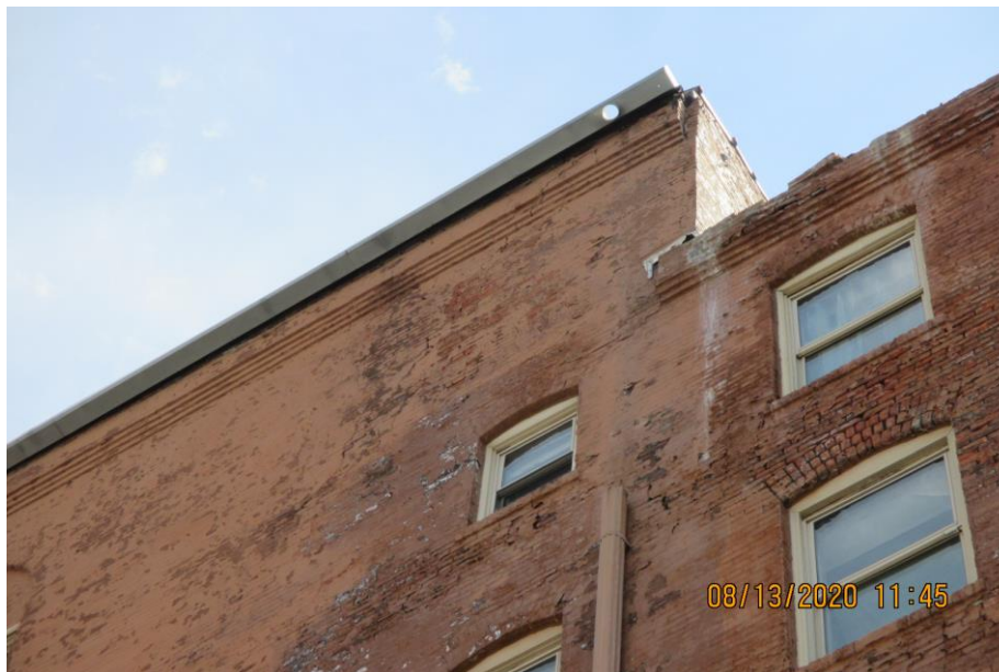
Photograph 2: August 2020 image of west elevation from City report. Note open mortar joints and masonry distress.
