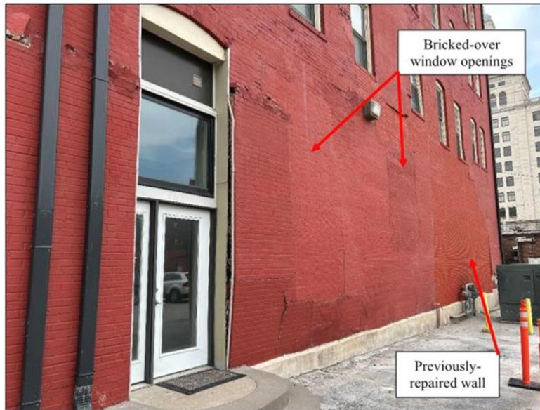
Photo 1 – Clay Brick Façade pulling away from Substrate
