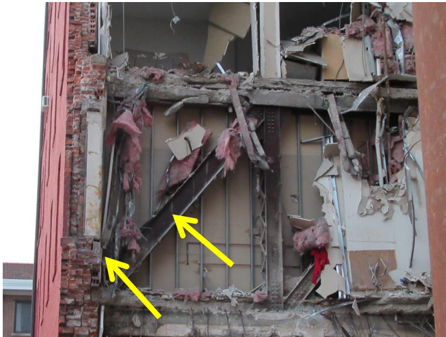
Fig. 20. Photograph of the northern extent of the collapsed portion of the Building taken June 4, 2023. Arrows indicate steel column (left) and truss (right).
