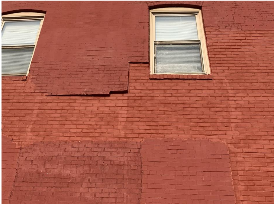
Photograph 27: Image from City file 23-30329. Note mis-aligned masonry at Pier E brick replacement locations.
