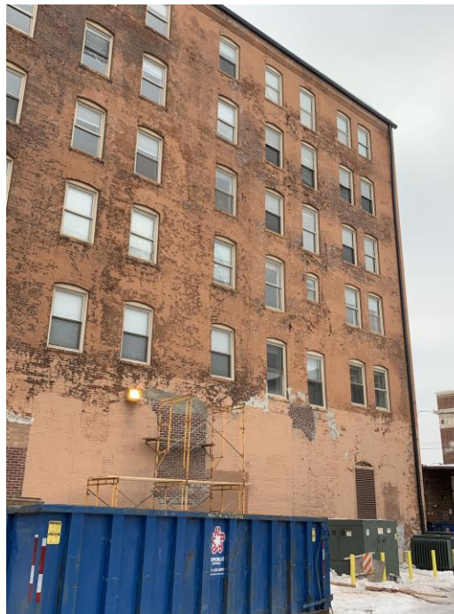
Photograph 6: 2021 image from City report. Note in progress limited repair work.
