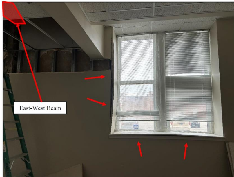
Photo 3 – Excessive Downward Pressure on Finishes
