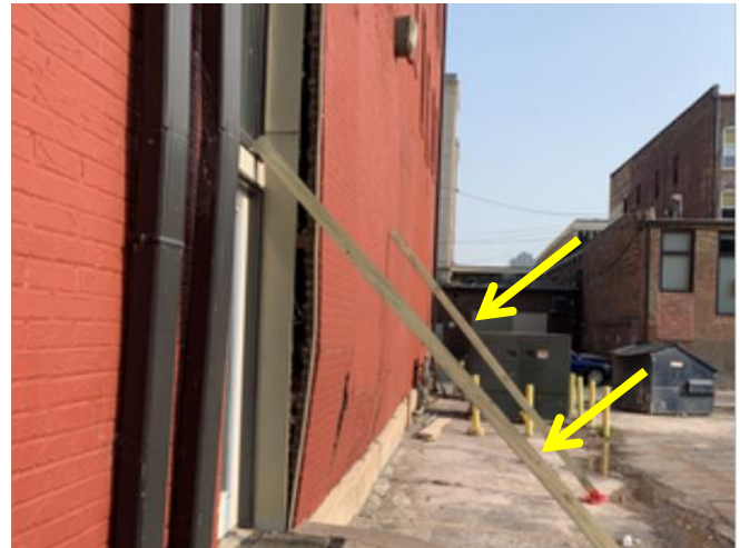
Photograph indicates area of bowing brick south of doorway. Note “shores” in place that do not appear to conform with SSE’s design.
