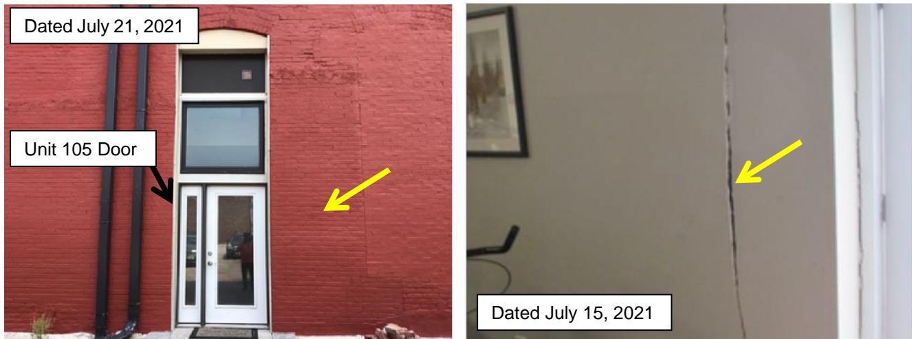
Fig. 30. Image of the west elevation adjacent the rear door, taken in July, 2021 (Ref: City Reinspection Report, Task ID: 21-42476). Yellow arrow points to apparent location of drywall crack at interior and exterior.
