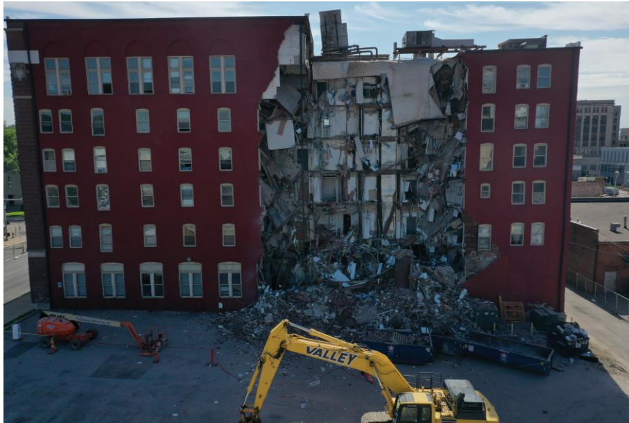
Photograph 35: Post collapse overview of west elevation from City sUAS.
