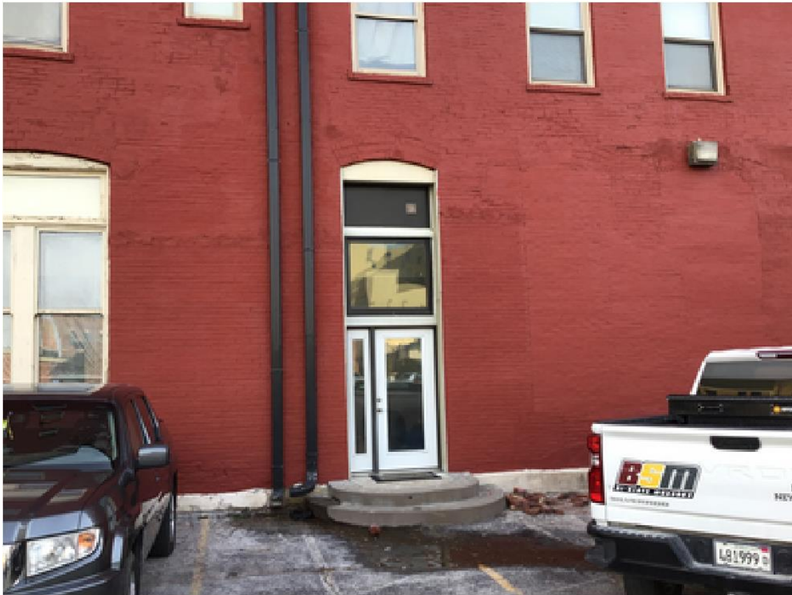
Fig. 31. Image of the west elevation adjacent to Unit 105 door taken on November 1, 2021 (Ref: City Report, Task ID: 21-64101).
