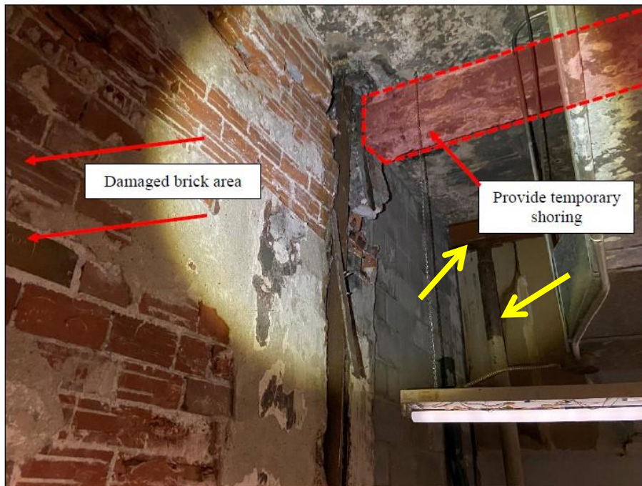
Photograph 32: Image and annotation from SSE February 2, 2023 letter. Yellow annotation (by WBG/SEI) denotes supplemental steel post and modern steel beam.
