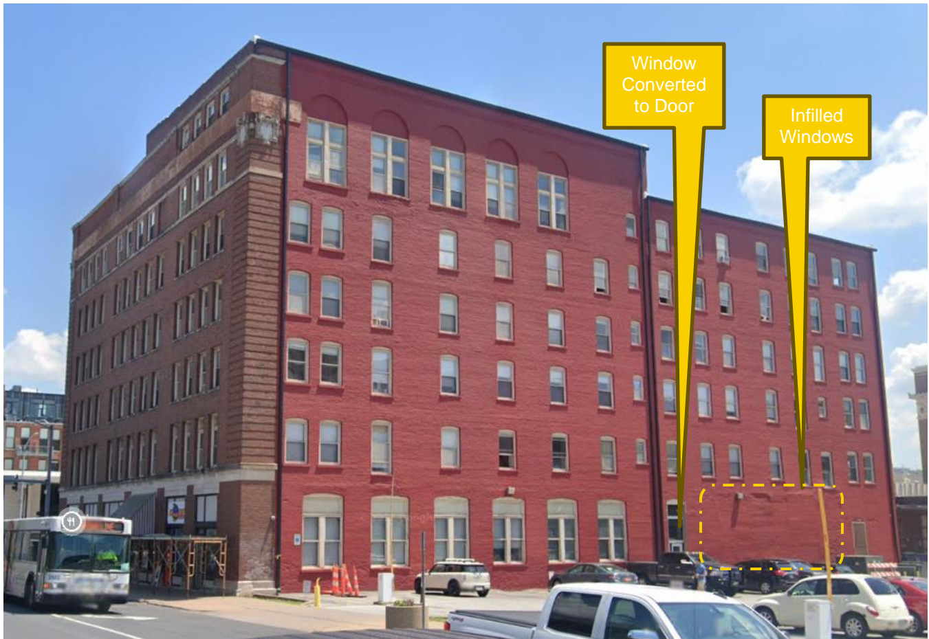
Fig. 4. Overall view of the west elevation of the Building (Ref. Google Streetview, dated June 2021). Annotation by WBG/SEI.
