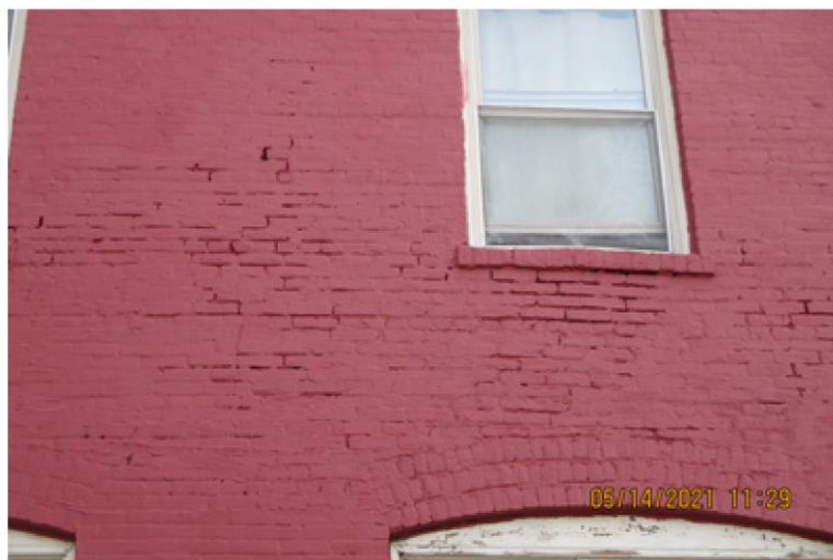
Fig. 29. Image of the west elevation indicating brick painting completed on May 14, 2021 (Ref: City Reinspection Report, Task ID: 21-9198).
