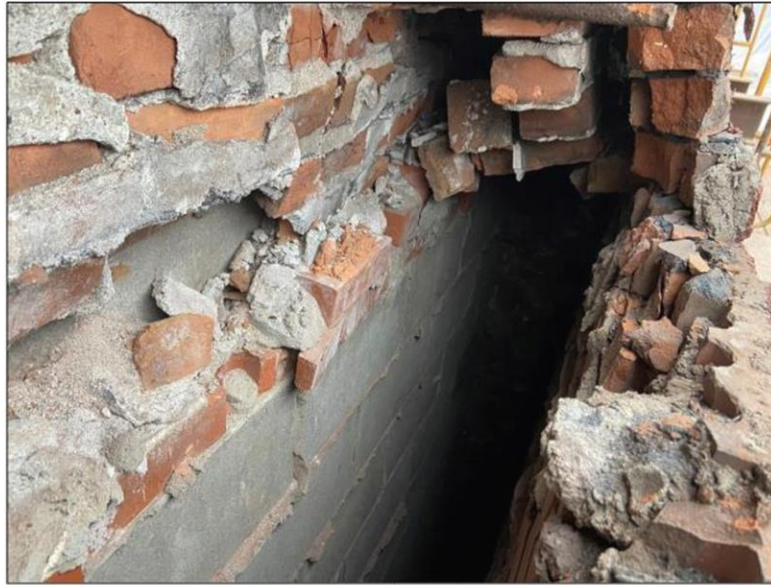
Photo 1 – Void between CMU and Clay Brick Façade
