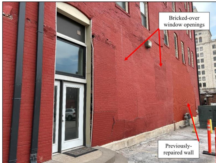
Photo 1 – Clay Brick Façade pulling away from Substrate
