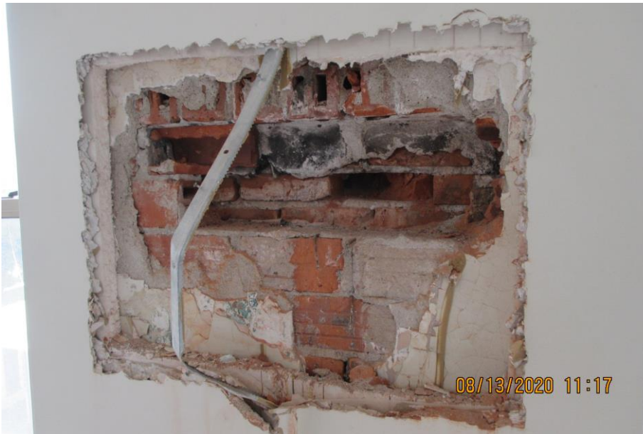
Photograph 8: August 2020 Image from City report. Note deterioration of brick masonry at interior wythes
