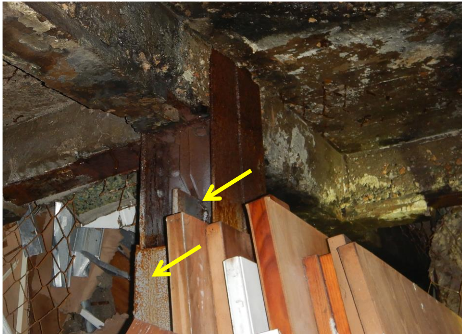
Photograph 33: Image and annotation by WBG/SEI of basement column. Note cover plate and vertical stiffener.
