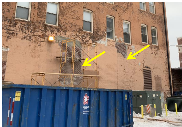
Fig. 27. West elevation photographs. (Ref: City Inspection Report, Task ID: 20-83090). Yellow arrows point to areas of apparent repair.
