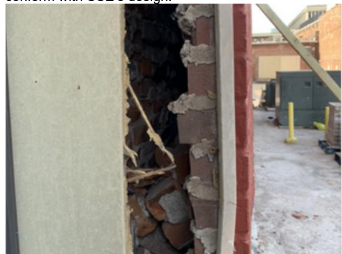
Detail view of bowing brick at south jamb of doorway. Note bricks accumulated in gap between wythes.
